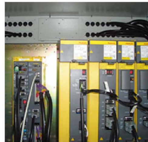
Water-proof fittings are mounted at the openings for wires to avoid invasion of oil mist.
